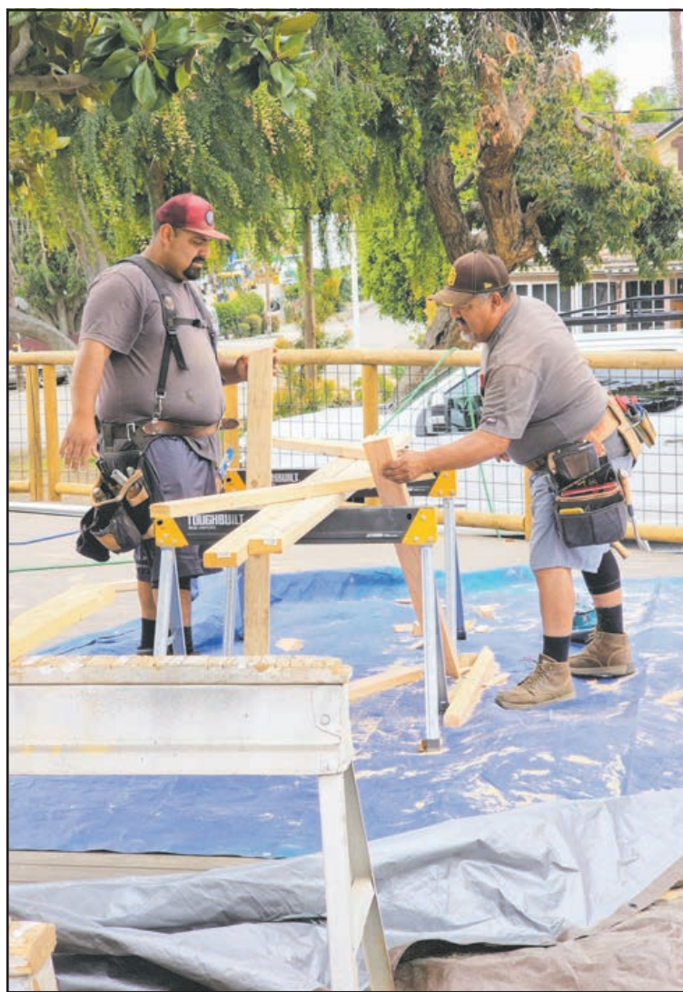
Domingo Chavez, right, and Arturo Chavez, Village News/David Landry photo a father and son team, work together to build the (now completed) ticket booth for Heritage Park located at the corner of Elder Street and Main Avenue. Domingo Chavez Construction Services has been servicing the Fallbrook community for over 30 years.
