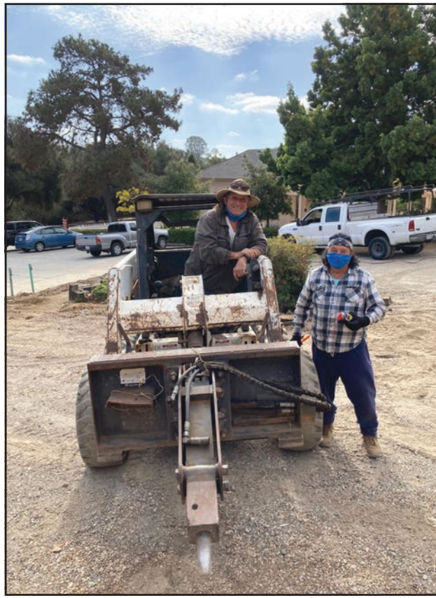
Art and Arthur Baeza of A & A Concrete paved the garden's brick-lined path, constructed a berm to prevent runoff, and installed a new walkway.
