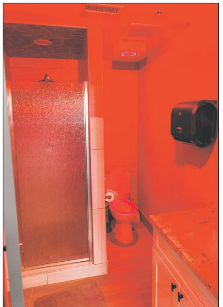
New red LED lighting illuminates a bathroom and other areas of Fire Station 2 alerting firefighters to an emergency call.
