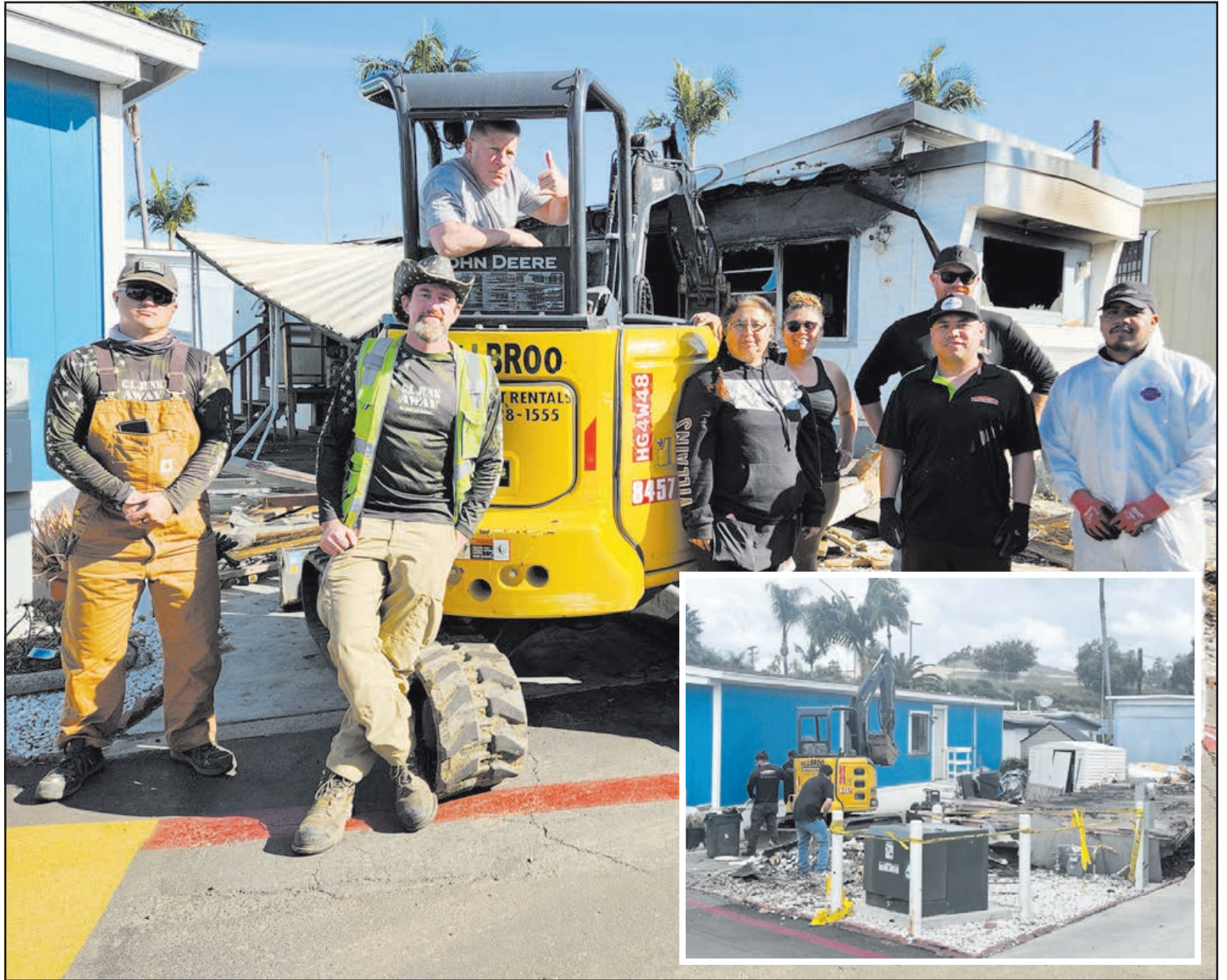
Local companies pitch in to help dismantle and dispose of the charred manufactured home that burned March 14, from left, Village News photo GI Junk owners Joshua Sperling and Blake Petricca; Tony Campbell from AC Investigations providing moral support, from an excavator from Fallbrook Equipment Rentals; Veronica Castillo, who lost her home; Lido Favela from Ace Party Rentals; ServPro owner Randy Vance, and ServPro employees Jose "Hong Kong" Torres and Robert Ramirez. [inset] Fallbrook ServPro team removes the remainder of the charred home and rubble, March 25. Village News/AC Investigations photo
