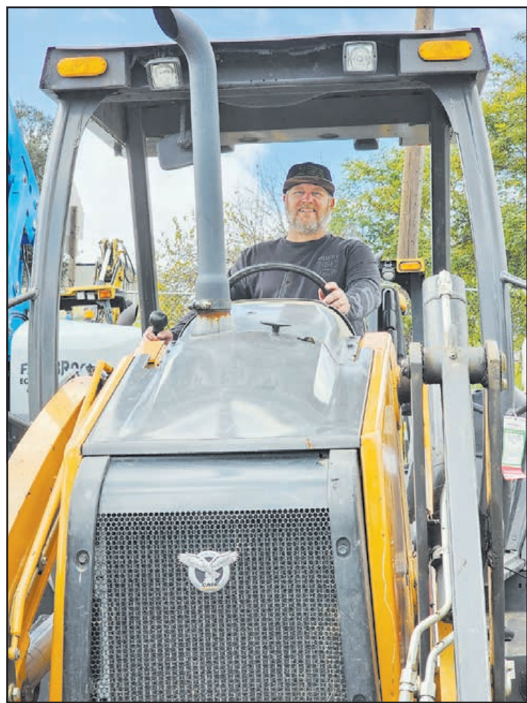
Brian Wagner picks up a tractor for his next assignment in Fallbrook. A heavy equipment operator foreman for a Local 12 Operators Engineers Union Contractor, he works on underground wet utilities. He has been doing this work for the past 27 years. His goal is to retire and enjoy life with his wife and travel some.
