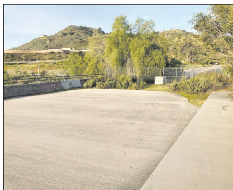
The west end of the bridge is blocked by bushes, trees and a fence.
