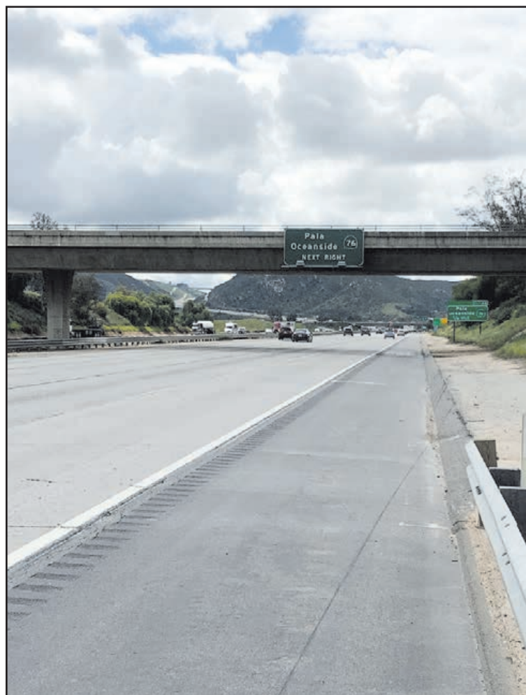
The bridge to nowhere crosses over Interstate 15 north of State Route 76. Village News/Derek King photos
