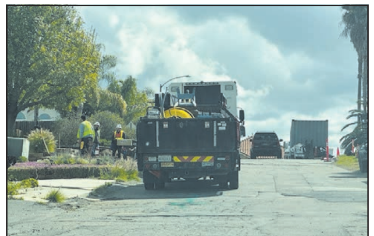
A gas leak at 948 E Elder Street in Fallbrook led to a road closure Friday, March 29.
