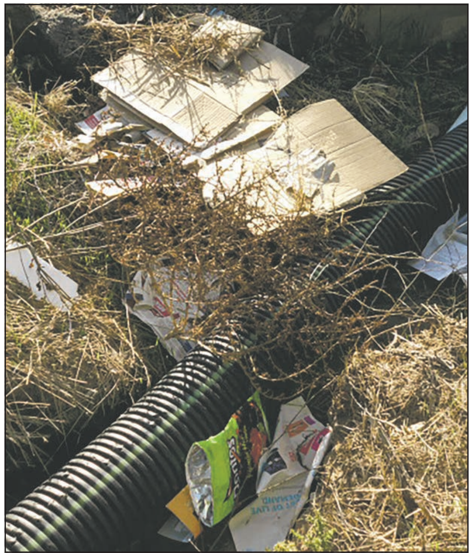
A drain is covered in trash on South Mission Road in Fallbrook.
