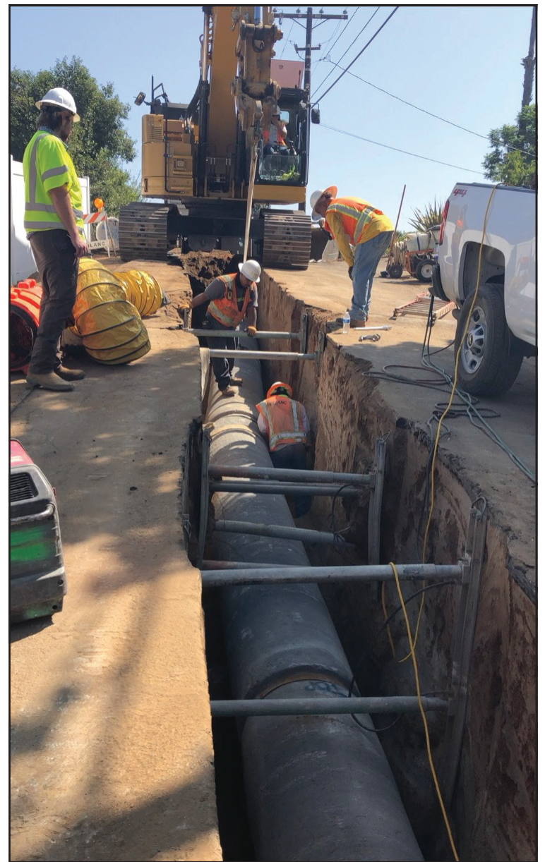
Crews work on the Santa Margarita River Conjunctive Use Project construction on Palomino Road. Village News/Courtesy photo
