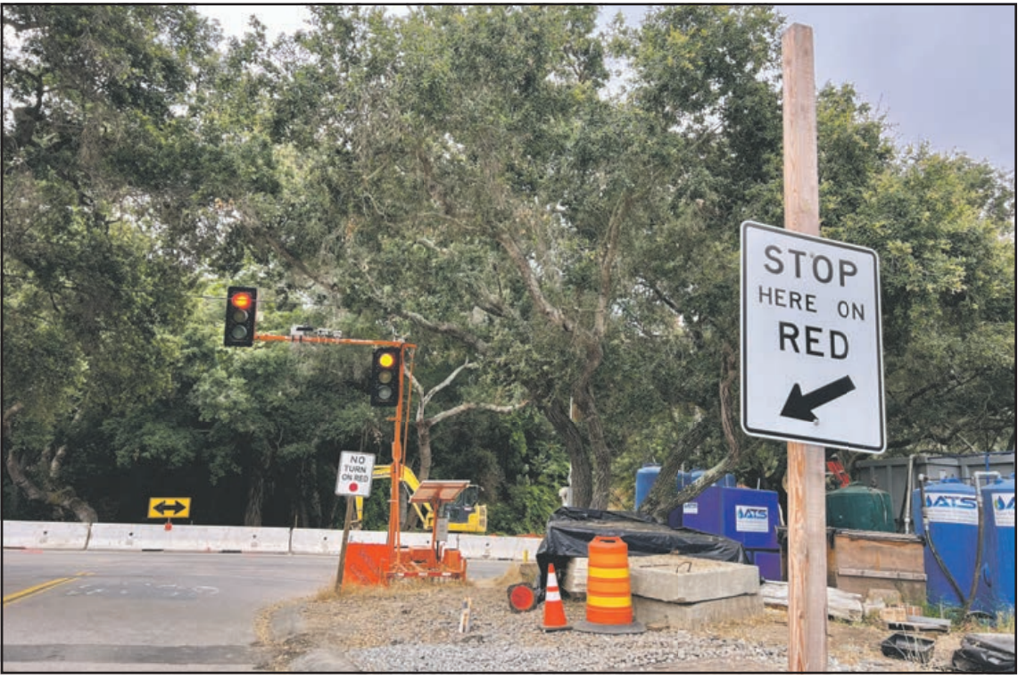
Traffic diversion at intersection of Live Oak Park Road and Gum Tree Lane where a new bridge is being built. Avalon Hester/Courtesy photo
